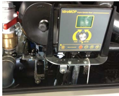
Computerized control unit.
