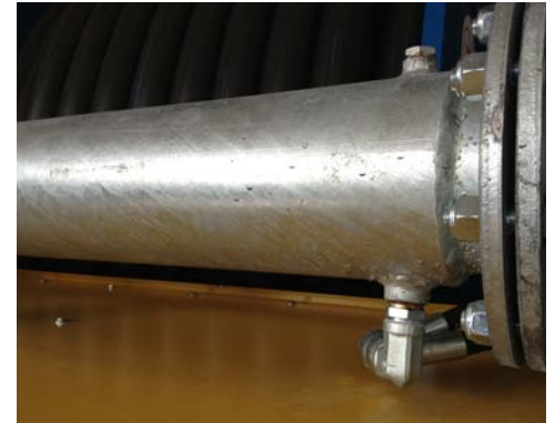
Oil cooling tank for hydraulic rewinding system instead of turbine.
